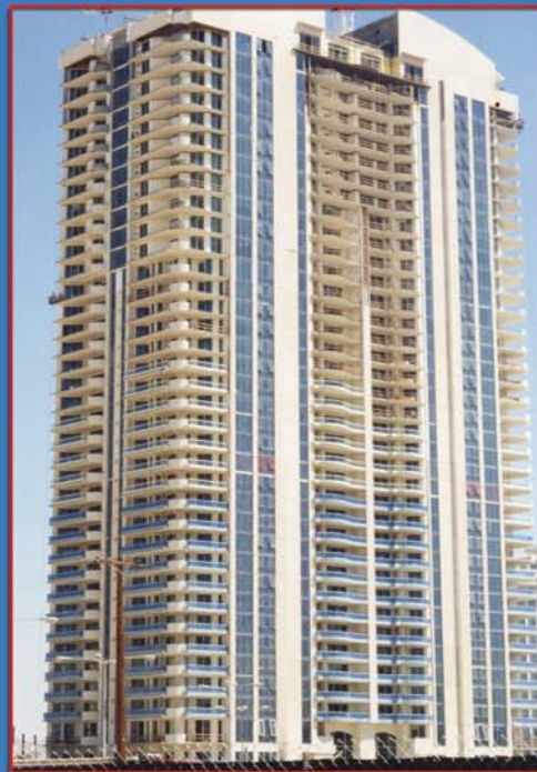
High Rise Building with Glass Cover™
